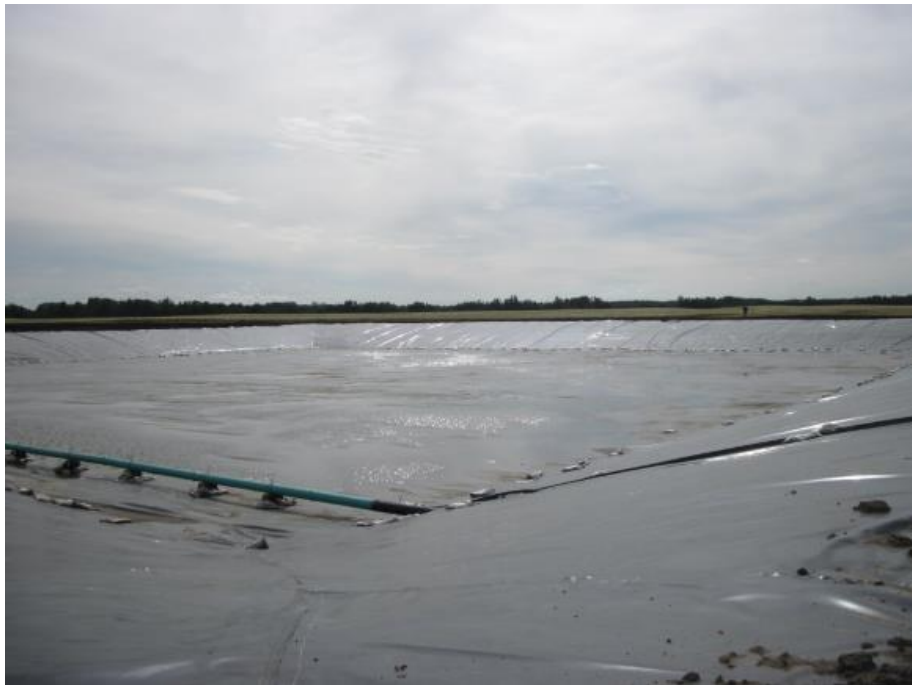
Newly excavated detention basin surrounded by cropland, northeastern / central section of the PA.
